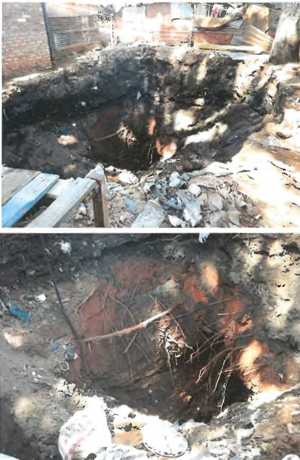
Figure 4: Sinkhole between the shacks in Makause Informal Settlement.
